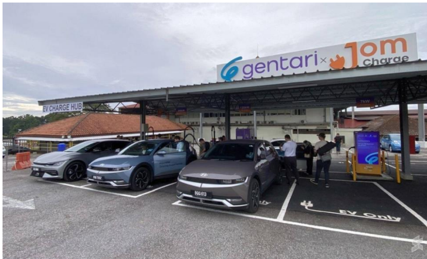
EV Charging Hub at Sunway Serene — Picture via SoyaCincau
